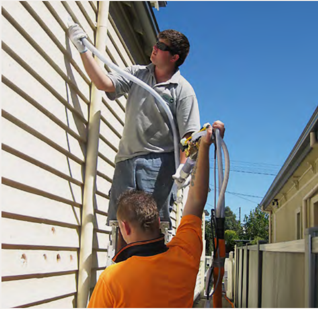
↑ Blow-in wall insulation is frequently installed through holes drilled in external weatherboards, which are then patched and painted.
